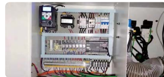
Electric box Simens & Omron brand Electric parts Delta brand PLC, CHNT switch
